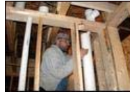
Plumber Kevin Waybright of Local 152 swabs plumber's glue to attach a coupling on a 4-inch plastic pipe at a residence hall that is being constructed at Potomac State College in Keyser, W.Va. Wesley Haines/Cumberland Times-News (Click for larger image)
