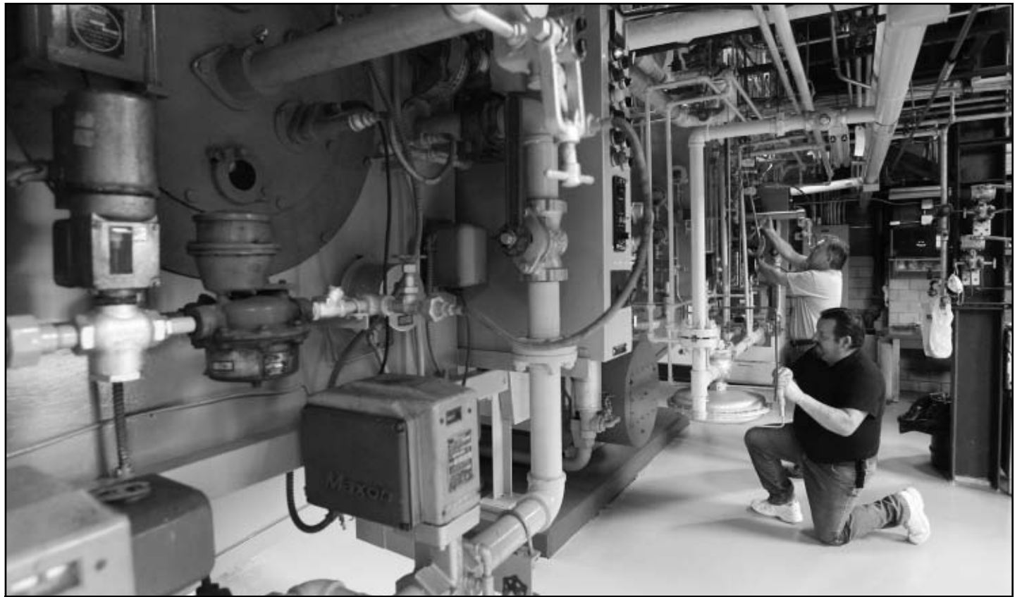
Leroy Staley and Bob Houston, both utility plant operators for Cal U, work on the boilers in the power plant on campus. Cal U's exemplary energy management program was recently highlighted in the PASSHE's 2006-2007 Green Report.
